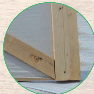
Detail Korrosion interlaced Papier
